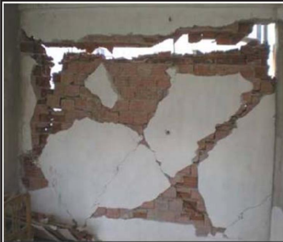
Kutahya Earthquake, Turkey May 29, 2011
