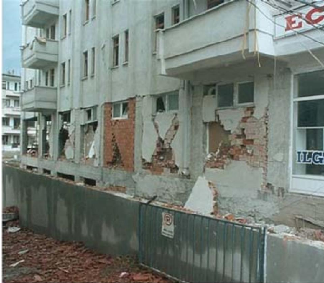
Duzce Earthquake - Turkey, Nov 12, 1999
