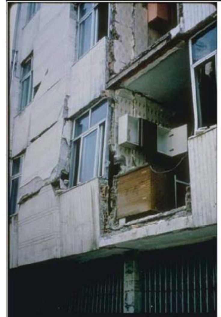
Manjil Earthquake – Northern Iran, June 21, 1990
